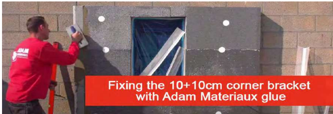
Fixing the LK PVC Premium 10x10cm corner to the corner of the facade with Adam Matériaux grey or white glue
