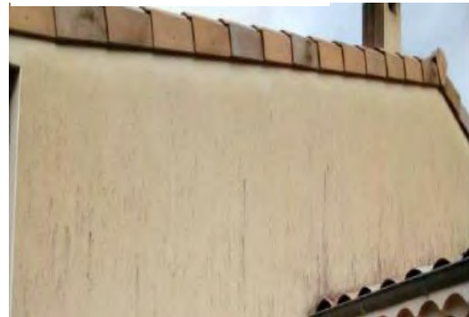
Badly placed roof overhang
