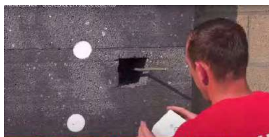
Electical cable passage through the EPS Adam Matériaux
