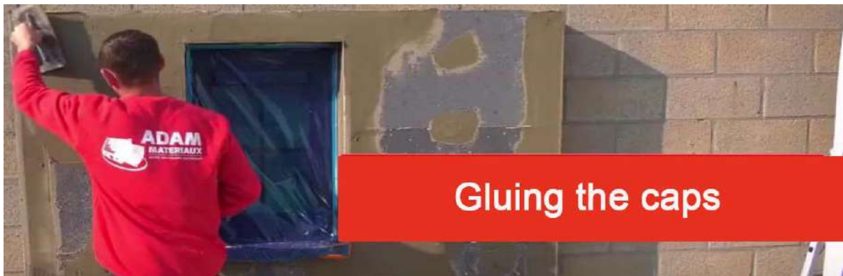
Applying “bandages” using Adam Matériaux gray or white glue to close the EPS caps placed to “drown” the fixing dowels.
